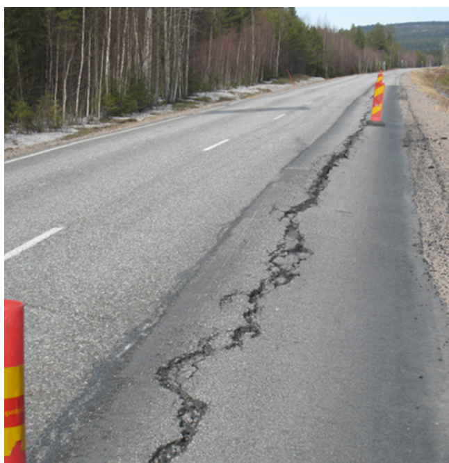
Differential frost heave between an old and a widened road section on road 934, Finland. (photo: Timo Saarenketo)
