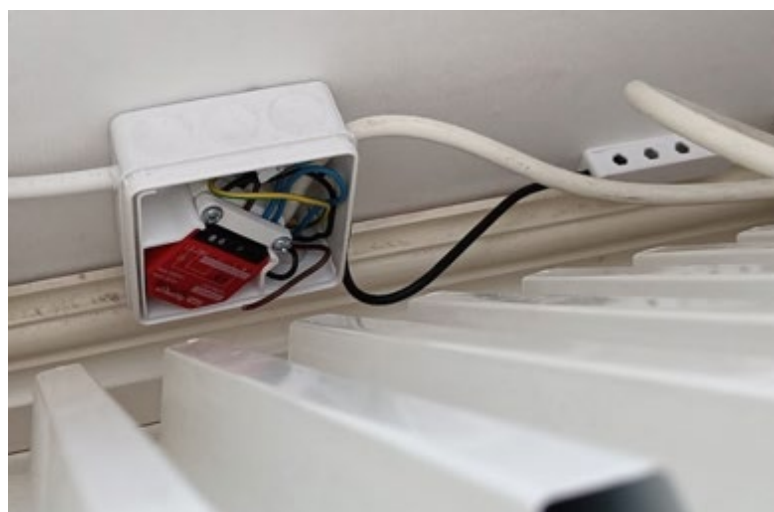
Figure 4: Shelly 1PM Gen3 smart relay installed
