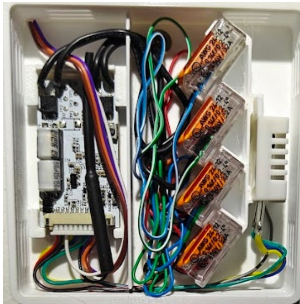
Figure 3: Shelly Plus Uni controller module installed
