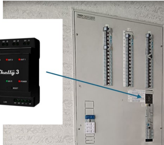
Figure 2. Shelly Pro 3 smart relay installed
