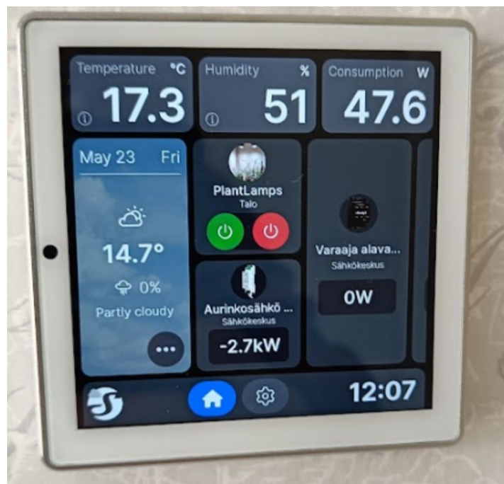
Figure 6: Shelly Wall Display units installed
