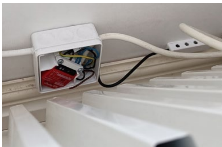
Figure 4: Shelly 1PM Gen3 smart relay installed
