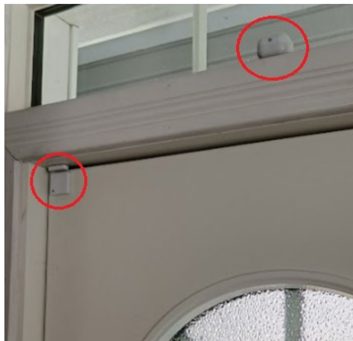
Figure 5: Door and motion sensors installed near the exterior door
