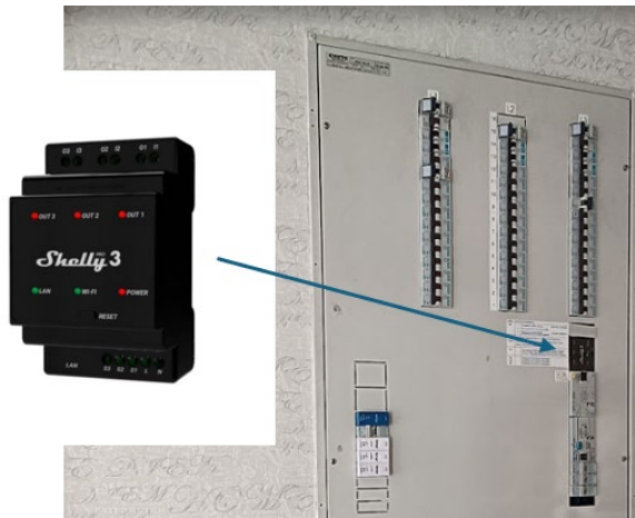
Figure 2. Shelly Pro 3 smart relay installed
