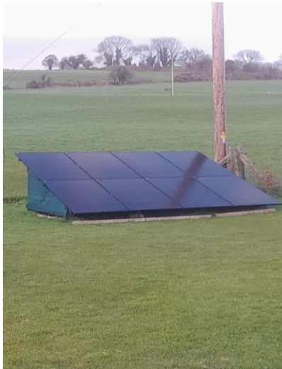
Figure 3. External Solar Panels at Kilworth House
